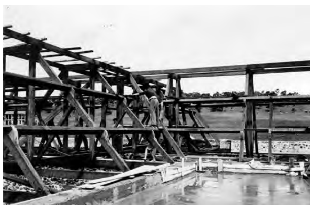
Bindoon Boys’ Town, building work, 1952. Photograph from Western Australia Government photographer collection. Source: State Library of Western Australia .
