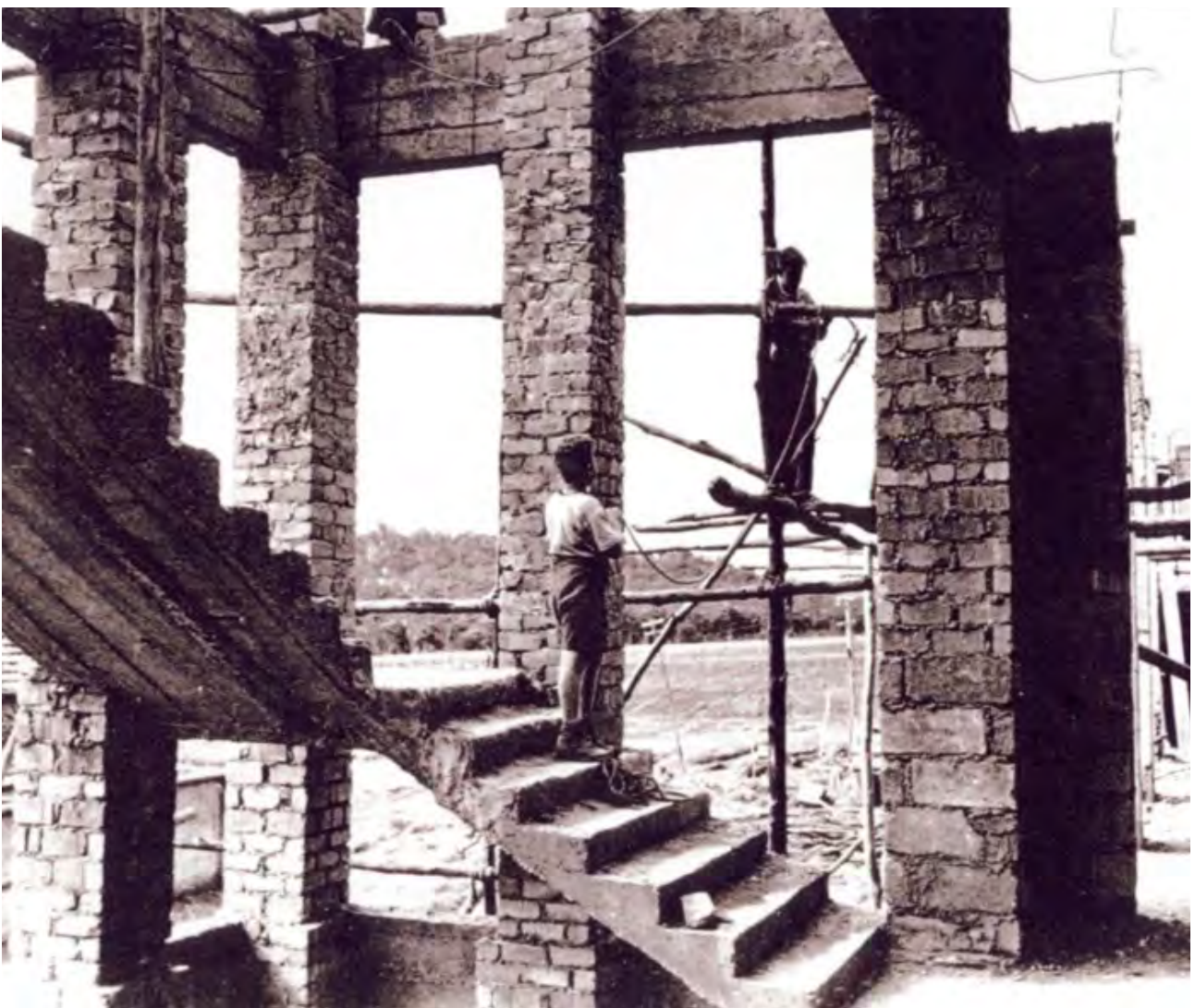
Bindoon Boys' Town, building construction, 1952. Photograph from Western Australia Government photographer collection. Source: State Library of Western Australia .
